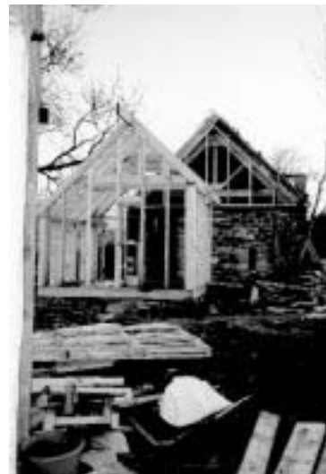
Bothy restoration at Wester Lawrenceton for Julia Hilton. Design by Edge Architecture and Design, Findhorn and built by Philip Stewart, Stuart Voder and Scott Gamble.
